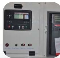
Control Panel & MCB
